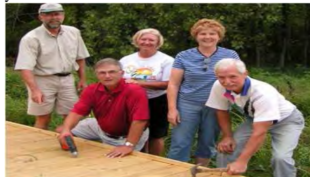
Washington CH Lions, Bruce Willis, Ray and Jana Deeks, Sue Willis, and Bob Mowry helped build a 600'+ boardwalk through local wetlands used for education and relaxation.
